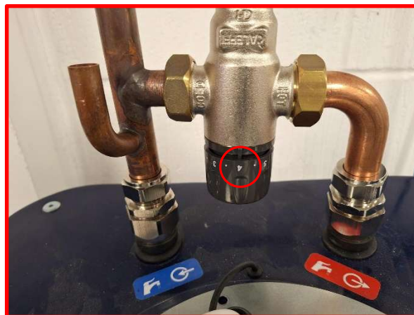
Figure 7: Mixing valve pipe set and valve set to position #4
